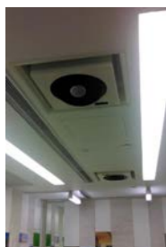
Figure 3.2.3 Rotating Fans (Source: Hong Kong Green Building Council)
