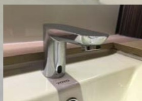
Figure 3.3.34 Hand Washing Sensor (Source: Hong Kong Green Building Council)
