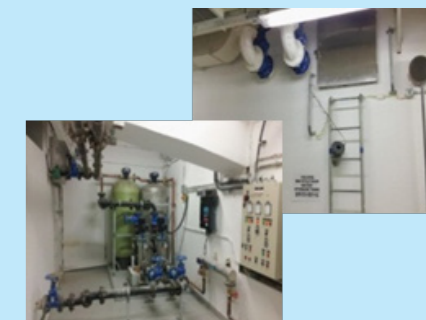
Figure 3.3.35 Rainwater recycling system
