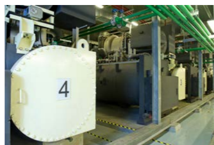
Figure 3.3.9 Air-conditioning System (Source: Kai Shing Management Services Limited)
