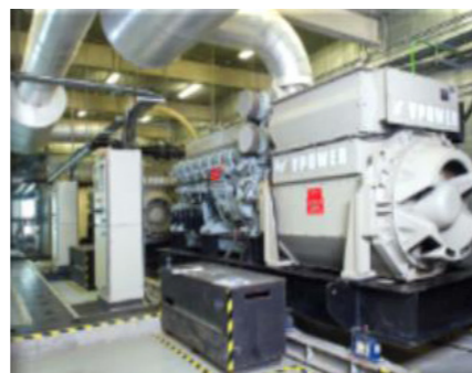
Figure 3.3.6 Electrical System (Source: Kai Shing Management Services Limited)
