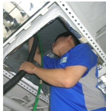
Figure 3.2.33 Air duct cleaning (Source: Hong Kong Green Building Council)
