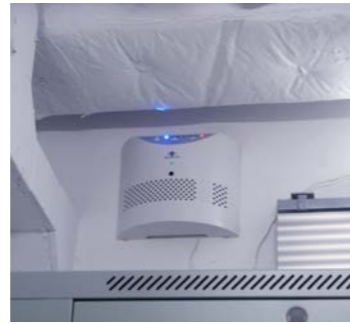
Figure 3.2.32 Air purifier in printer room (Source: Hong Kong Green Building Council)
