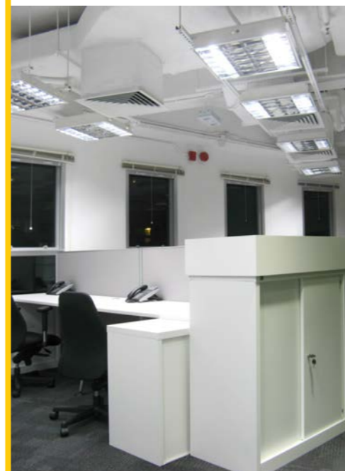
Figure 3.2.23 Hong Kong Green Building Council Office Interior (Source: Hong Kong Green Building Council)
