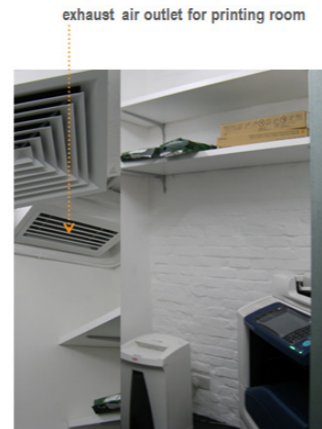
Figure 3.2.35 Location of exhaust (Source: Hong Kong Green Building Council)
