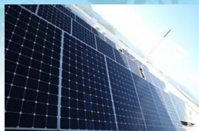
Figure 3.3.1 Photovoltaic panels installed on roof (Source: Hong Kong Science and Technology Parks Corporation)
