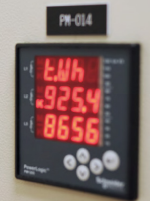
Figure 4.1.33 Smart Metering (Source: Business Environment Council)
