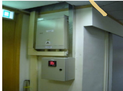
Figure 3.3.24 Power analyser (Source: Business Environment Council)
