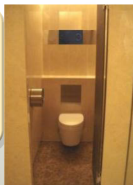
Figure 3.3.33 Dual flush sensor (Source: Hong Kong Green Building Council)
