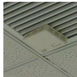
Figure 3.3.26 Air-conditioning control (Source: Jones Lang LaSalle)
