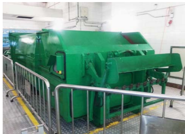
Figure 4.1.17 ICC in-house waste compactor (Source: Kai Shing Management Services Limited)
