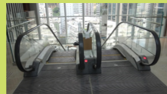
Figure 3.3.5 Escalator with infra red sensor for energy saving
