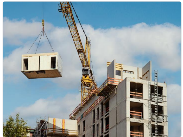
Figure 99: Adoption of MiC Lifting and installation of MiC modules on construction site.
