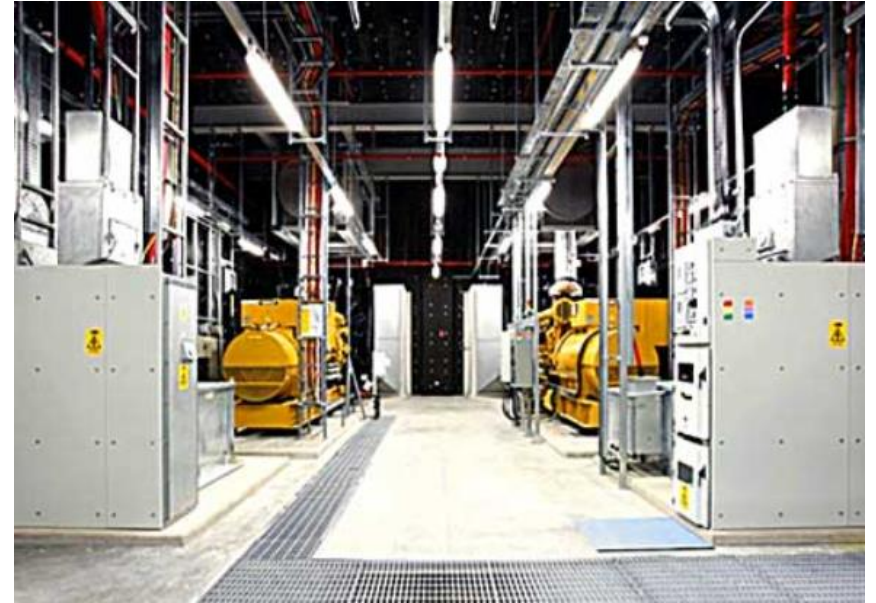
Backup Generators | Data Center
