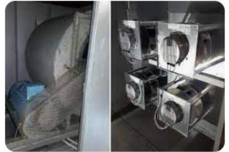
Old AHU Refurbishment with EC Fans
